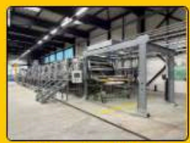
2012 Benninger / Kusters LT-TB-AR Pre washing installation
