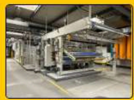
2004 Monforts MONTEX 6000-10F TWIN-AIR Stenter line
